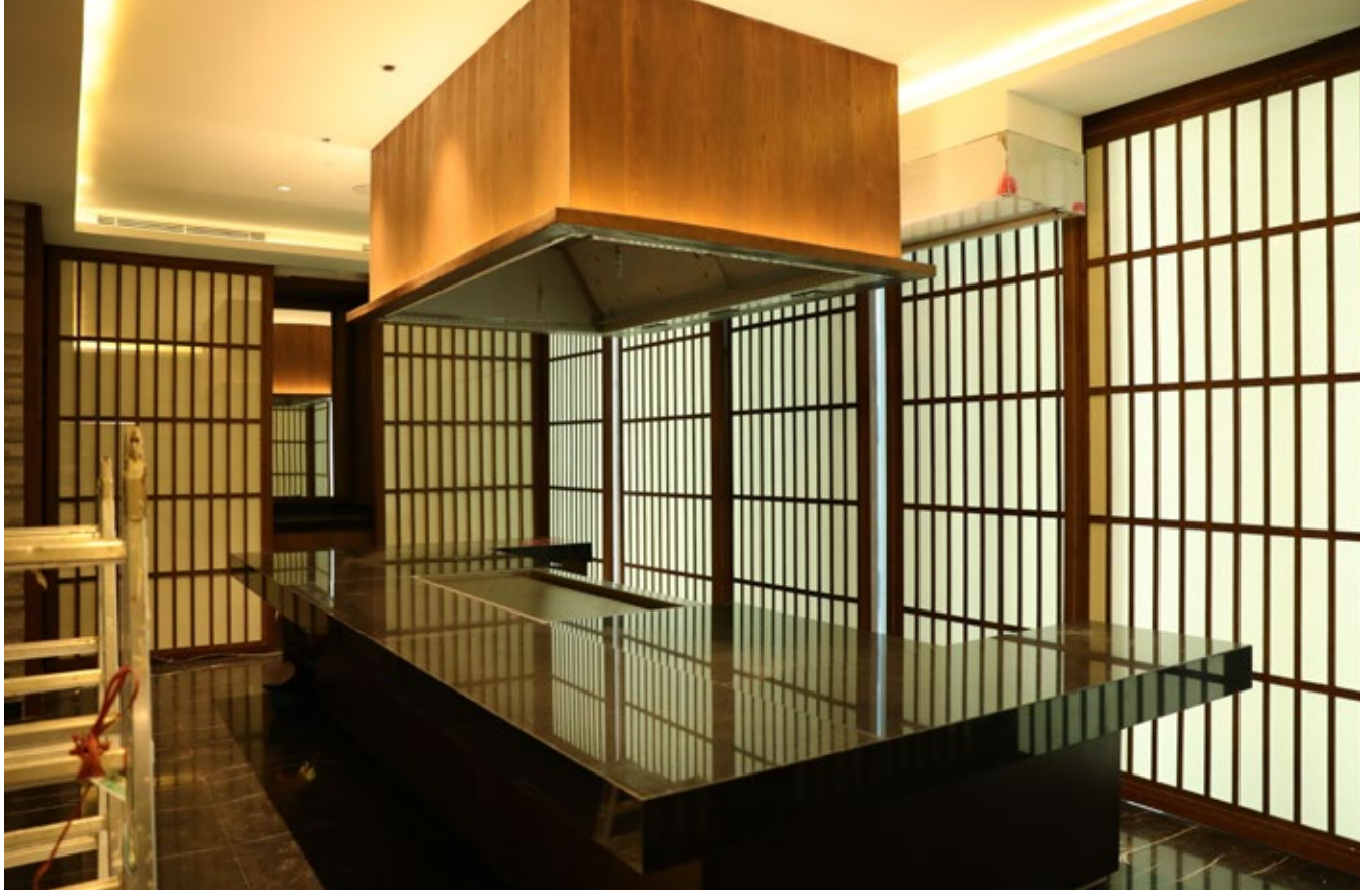
Teppanyaki Dining Room will test exhaust system on mid August. Furniture will be installed on end of August.
