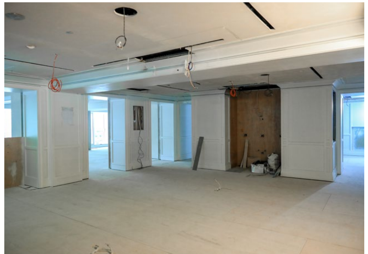
Lumen Meeting Room: ME and finishing work is 70% done. 7 meeting rooms, billiard, board room, music room, and Lumen bar will all be on level 2.
