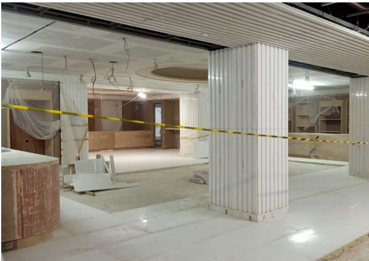
Gourmet Market: ME work, interior, and Bianco Dolomiti marble installation is 70% done.
