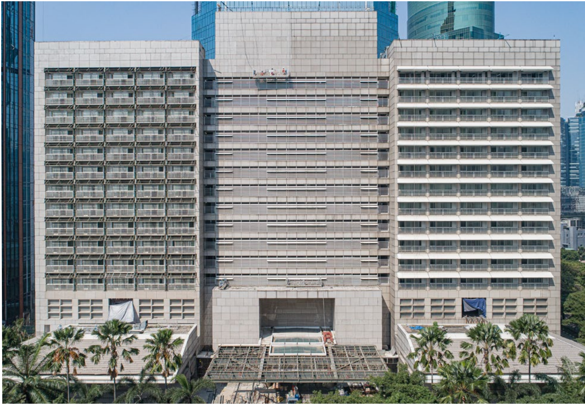
Hotel Facade: Lobby canopy and wall artwork is on progress. Bronze fin will be installed. Main Lobby water proofing is 40% done.
