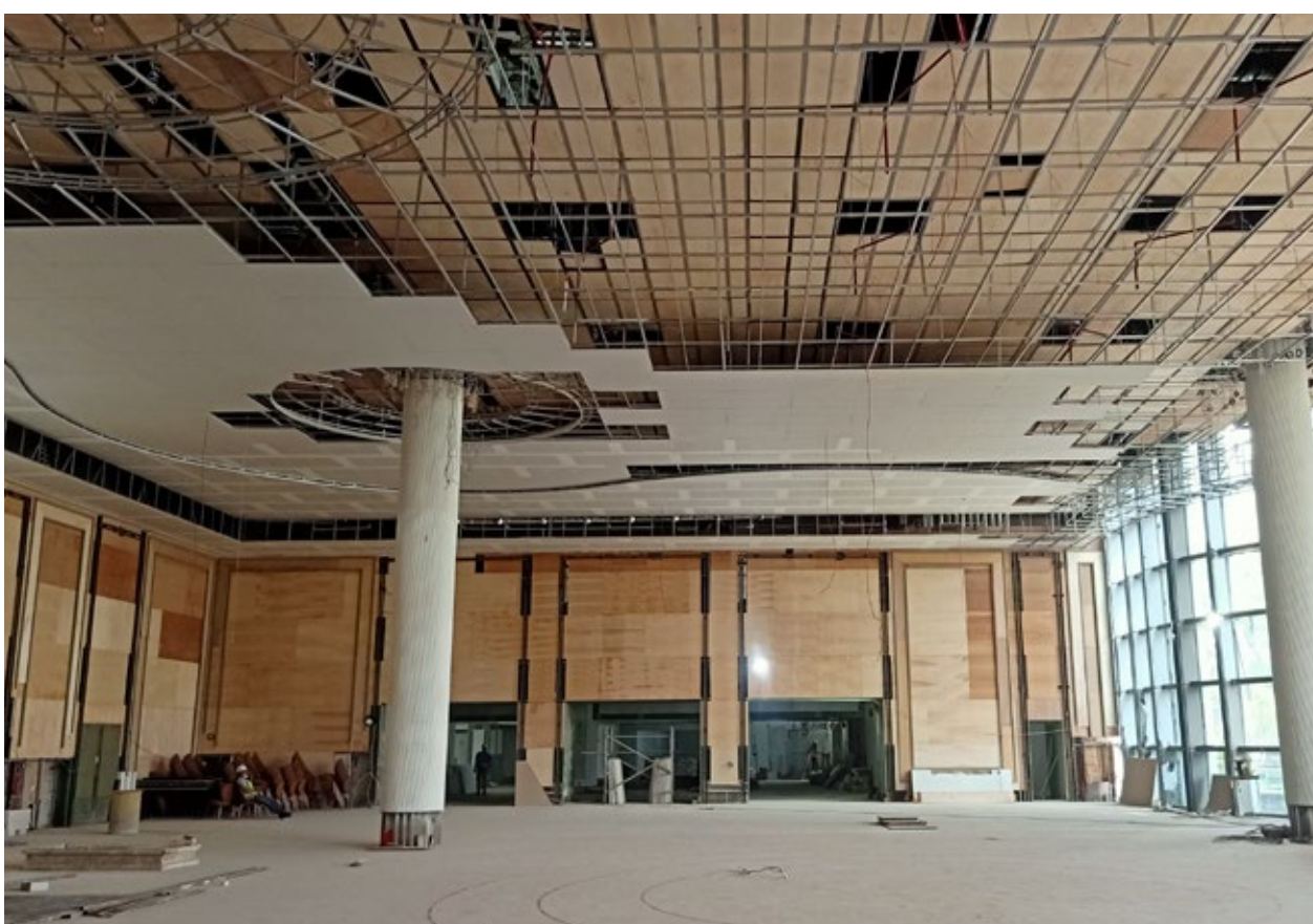
Grand Ballroom: Ceiling and chandelier is 70% done. Chandelier is made by Lasvit and will be installed on February 2022.
