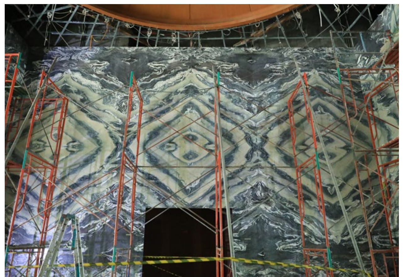
Lobby Concierge: By the end of December 2021, all Callacata Carrara marble are installed on lobby area.
