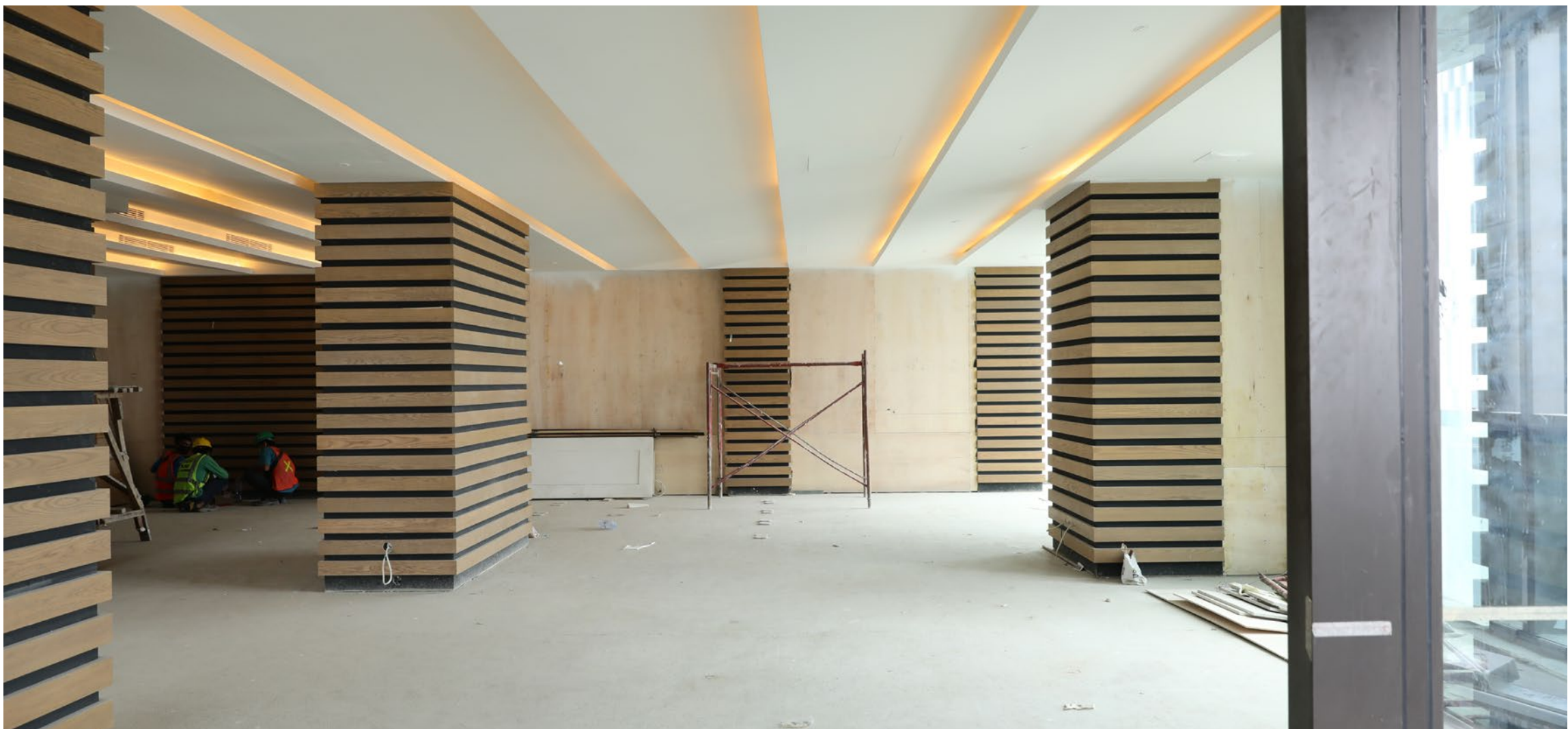
Level 23 is progressing smoothly. The timber walls have been installed, paint finishes will be applied to the ceiling soon, and parquettes will be installed in mid September 2021.
