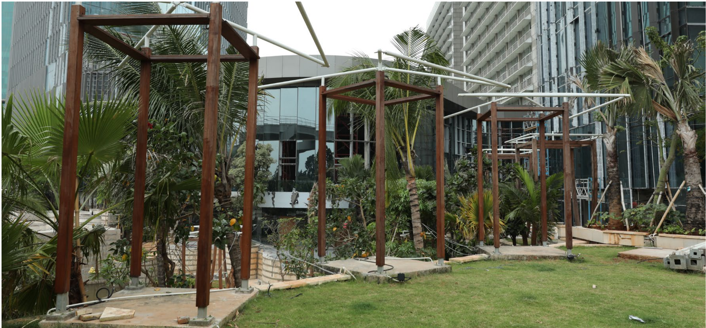
Landscape feature installation including gazebos, water pond, pavilions, and beautiful pavings is 60% done.
