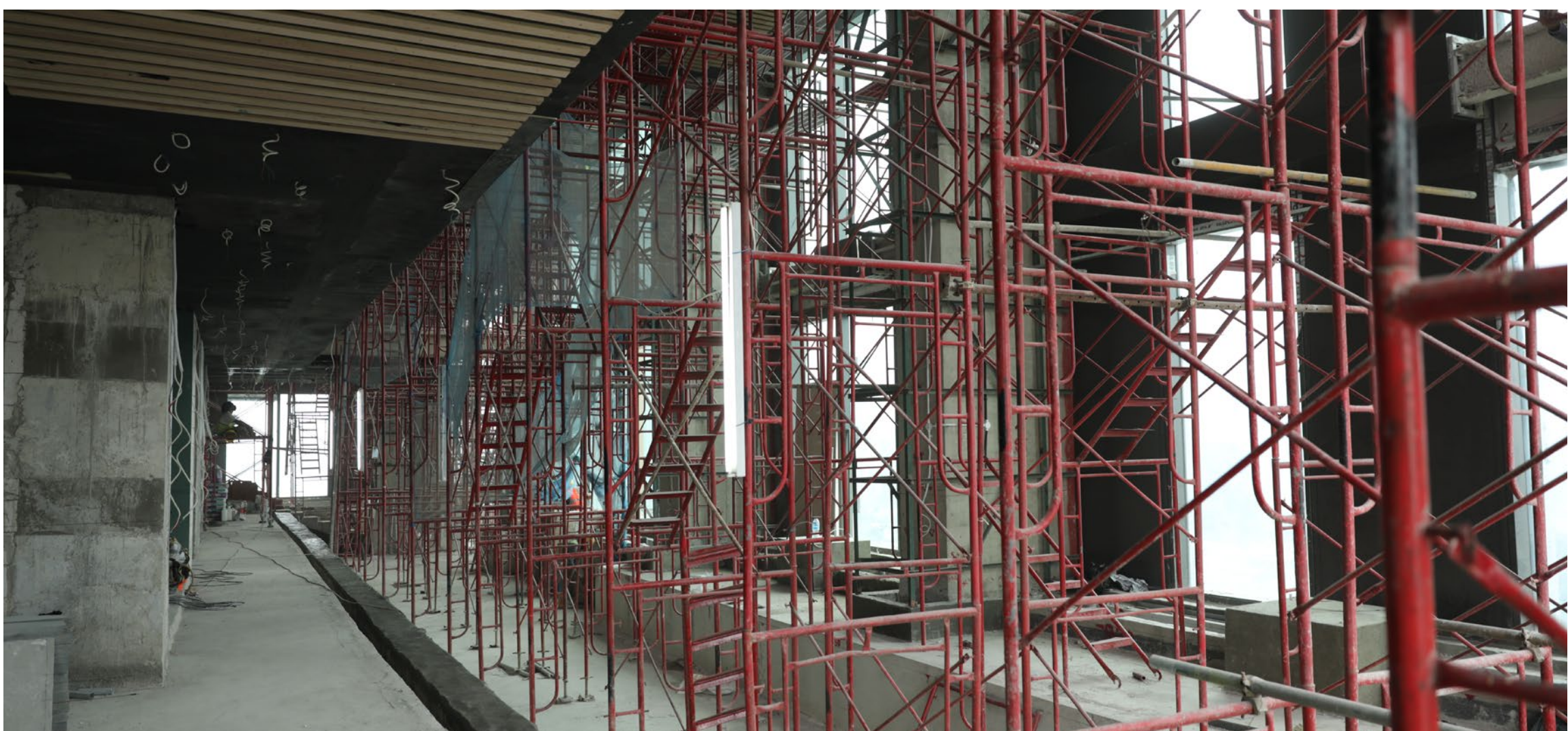
The construction of the indoor swimming pool on level 22 is underway. Swimming pool 'Bizaza' mosaic is currently on installation (70% done).
